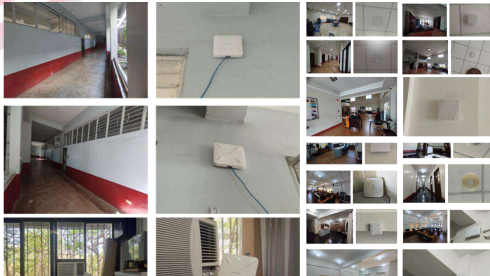
Figure 43. Installed Access Points
